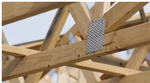
Standard gang nailed trusses must not be visible from the exterior
